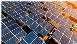
Photovoltaic (PV) Panels
