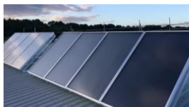
Solar Thermal Panels
