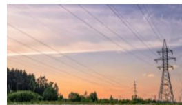
Power Lines and Support Structures
